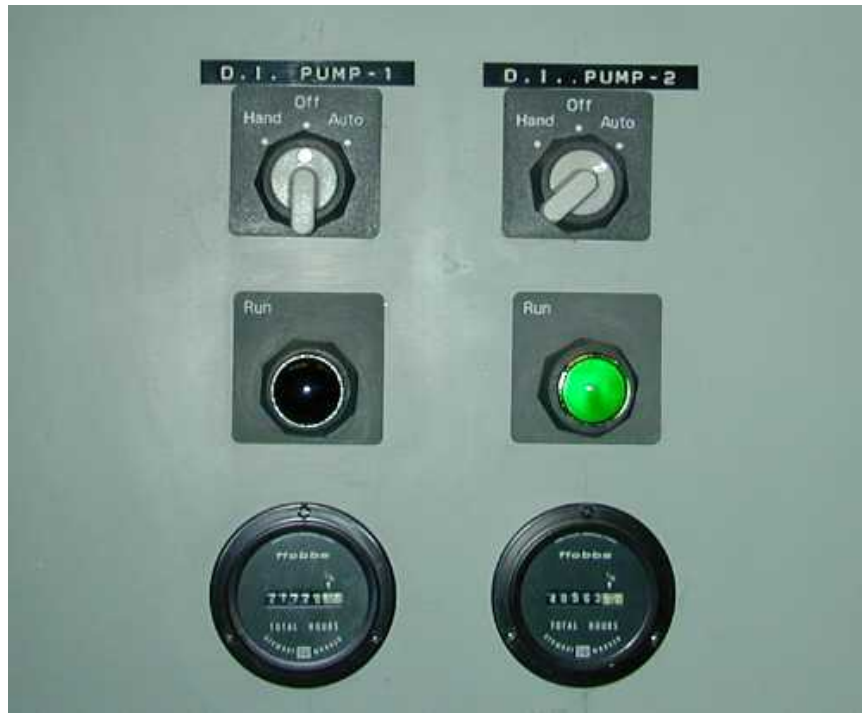
FIGURE 4. Deionized water pump control panel.
