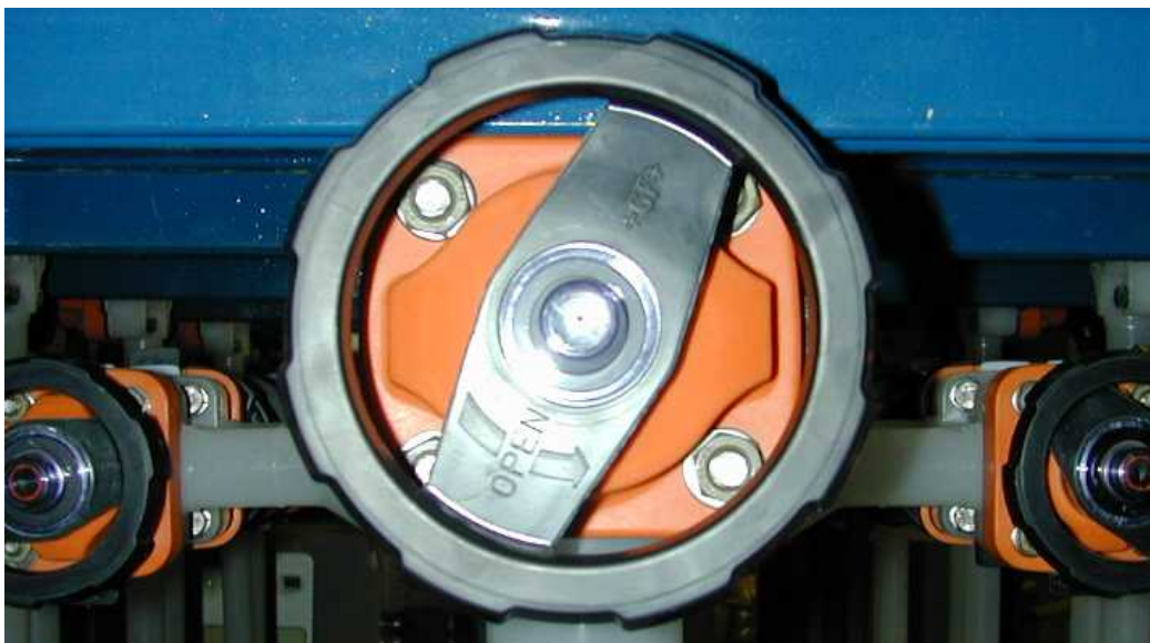
FIGURE 5. Deionizing polishing bed bypass valve, PVmb.
