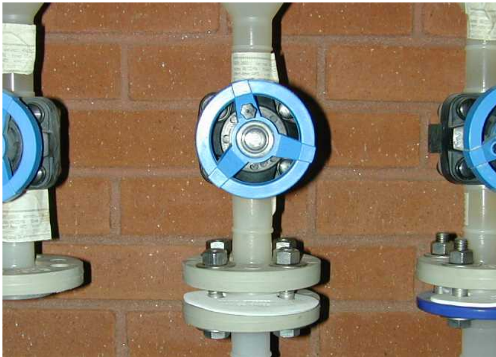
FIGURE 13. Deionized water output valve.
