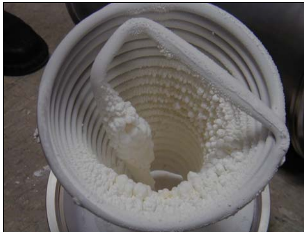
Figure 2-10 Cooling Spiral tube with Ammonium chloride ( \text{NH}_4\text{Cl} ) deposit
