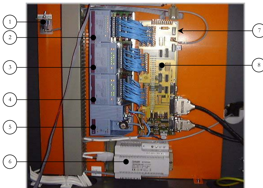
Figure 5 Servo drive control unit
